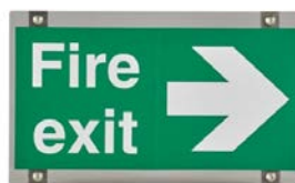
Emergency Exit Sign
